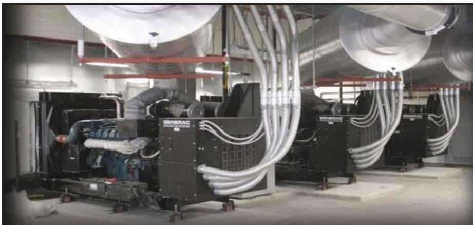
This 3 x 500 kW Diesel MPS installed at Doctors Hospital, Edinburg, TX, provides redundant power for critical loads. The MPS provides all the benefits of parallel generation in a simple, single-source system that allows end-users to quickly and easily add units as additional power is needed.
