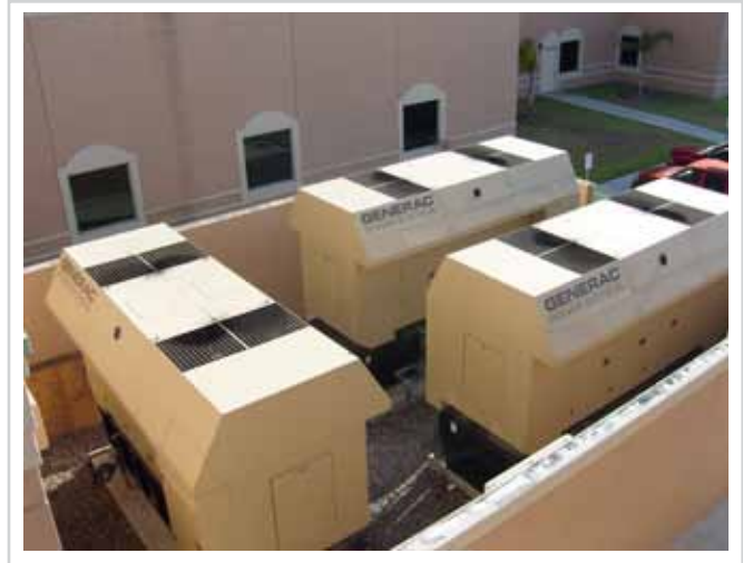
At Doctors Hospital, Generac's modular platform kept all critical systems operating for 13 straight days.
